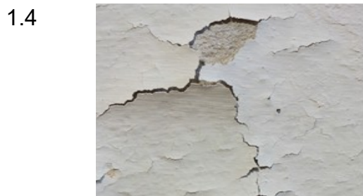
(A) Flaking or peeling✓
