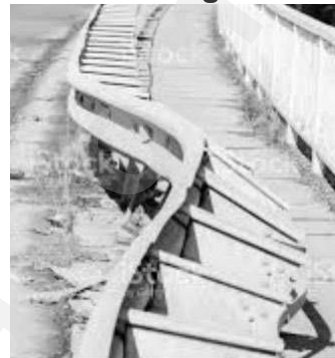
Barrier after being crashed into
