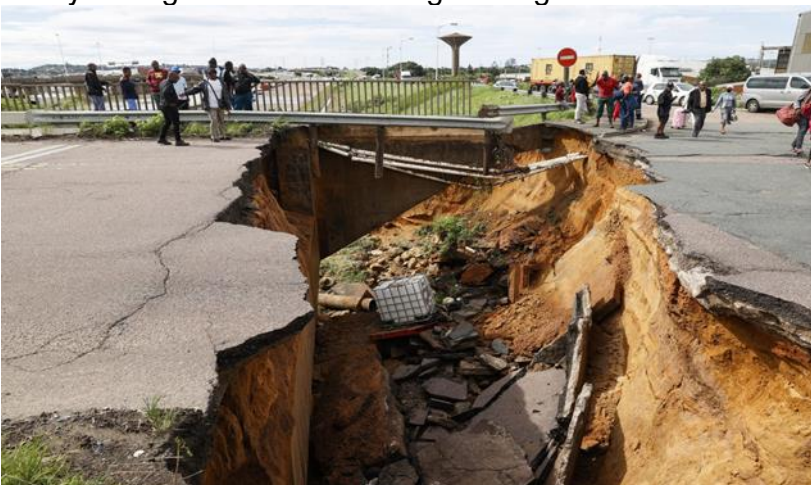
Figure 3.5: Damaged roads due to flooding in KZN
